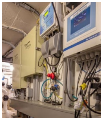
My quest for water-quality perfection began on the service route, and has led to years of experimentation, adaptation and implementation.
