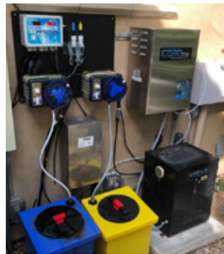
Correct Ozone installation (without use of bromine). Photo: Liquid Paradise Pools, Los Angeles
